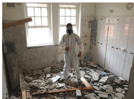
Over the past decade every single bathroom at TAS has been replaced at a cost of almost $750,000
